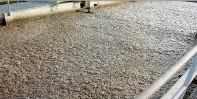
End biological basin (activated sludge)
