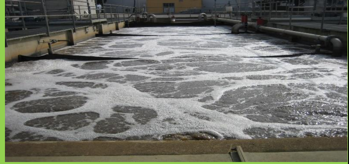
End biological basin (activated sludge)
