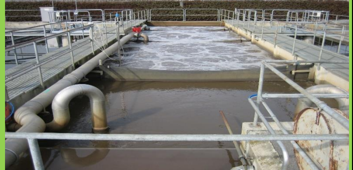
Biological basin (activated sludge)
