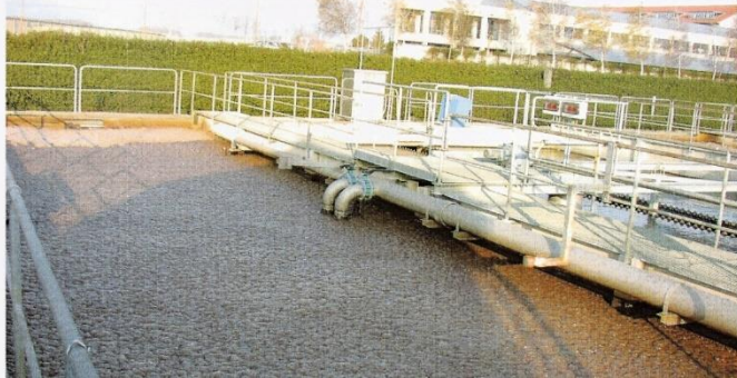
Biological basin (activated sludge)
